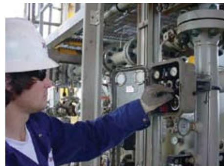
Blake Bowling adjusts the system pressure on a production separator on a Merit Energy platform.
